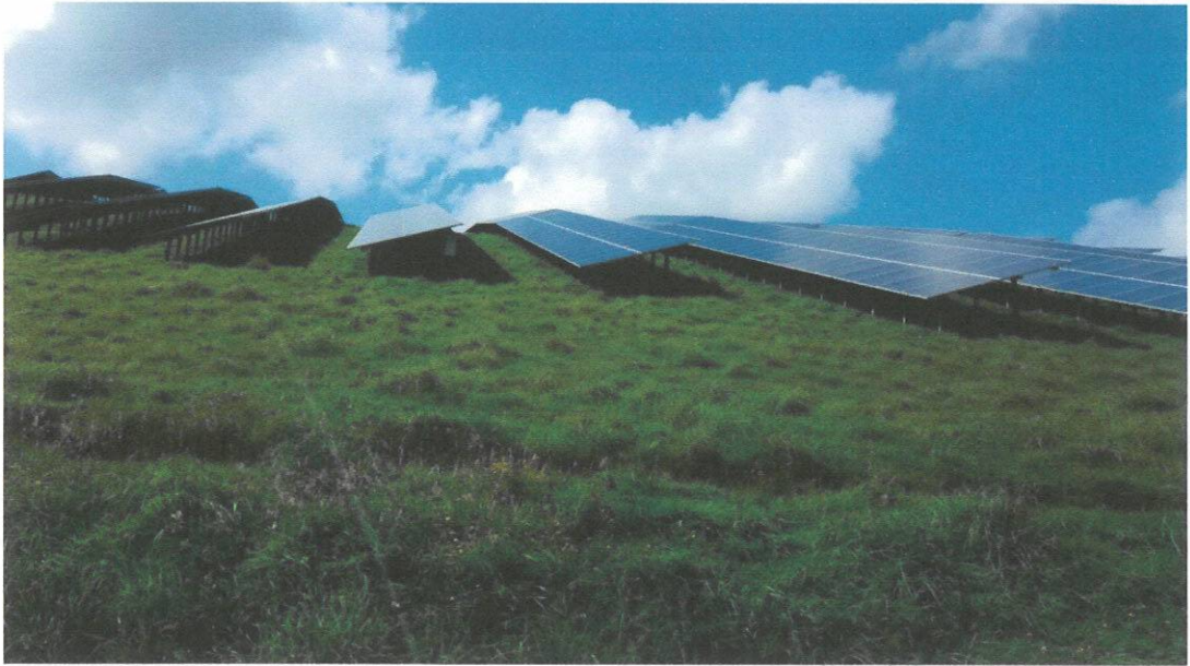
Trequite – Photograph of the ground beneath the panels at this site that has been in operation since 2013.
