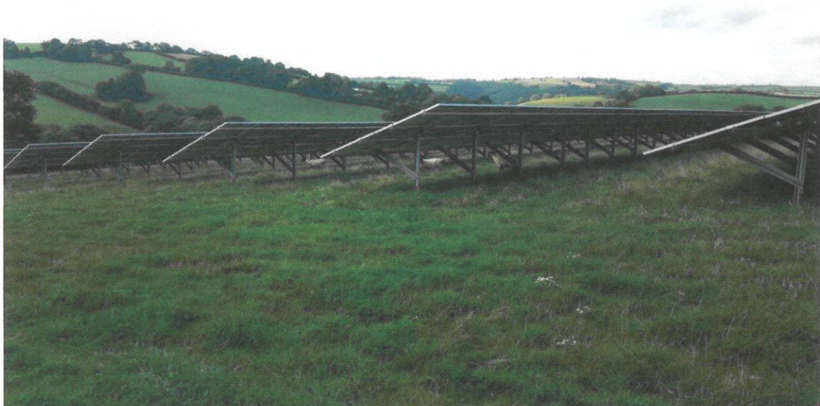
Insert 1-1: Photographs of an operational Solar Farm in Trewidland, Cornwall, UK. (Photographs taken by Tobin Consulting Engineers during a site visit in September 2015)
