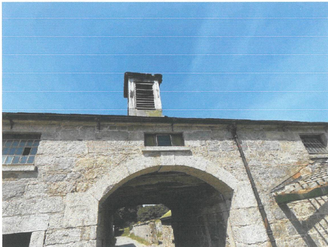
Fig 5 View of carriage arch and belfry. Belfry needs re-slating and repair.
